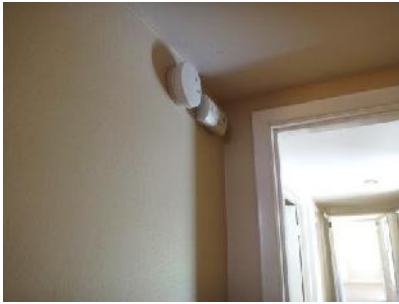
Improper detector mounting
